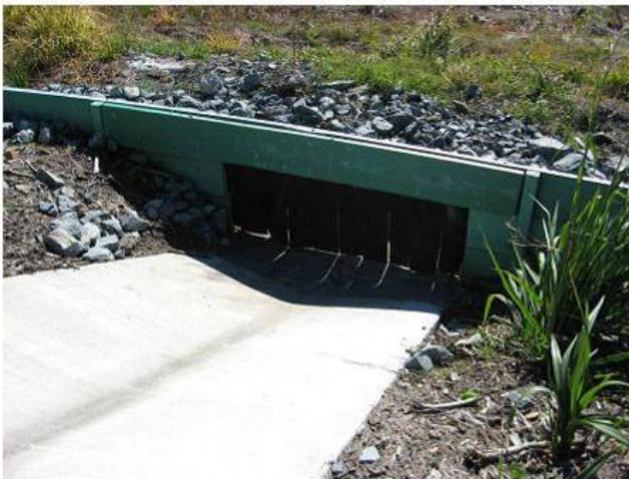
Figure 9.1.18 Concrete batter chute channelling water through the frog fence. Rubber flaps were installed to minimise frog access.
