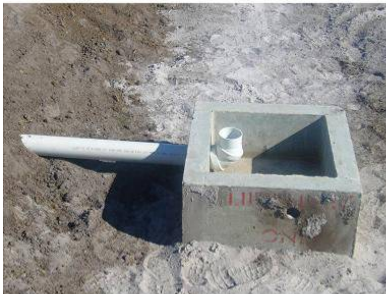
Figure 9.1.24 uPVC twister used to control water level in ponds.
