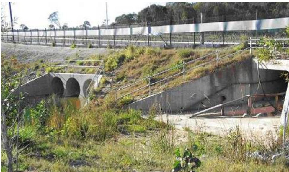
Figure 9.2.7 Kuraby Bushland entrance to an underpass and the wet culverts opening into an artificial pond. The fauna exclusion fence is also visible above the culverts (Bond and Jones 2006).
