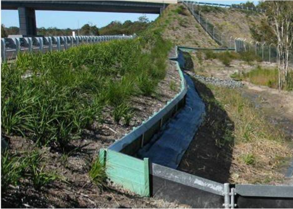
Figure 9.1.17 Backfilling behind frog fences has caused drainage problems.
