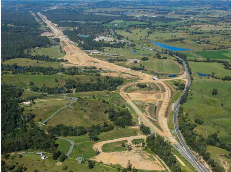
Progress of final earthworks at the northern end – showing the Woondum connections to the existing Bruce Highway (May 2017)
