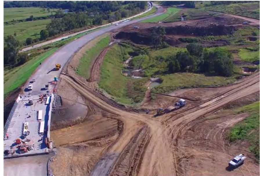
Progress of final earthworks at the northern end mid-June – showing the Woondum connections to the existing Bruce Highway and the Woondum interchange bridge
