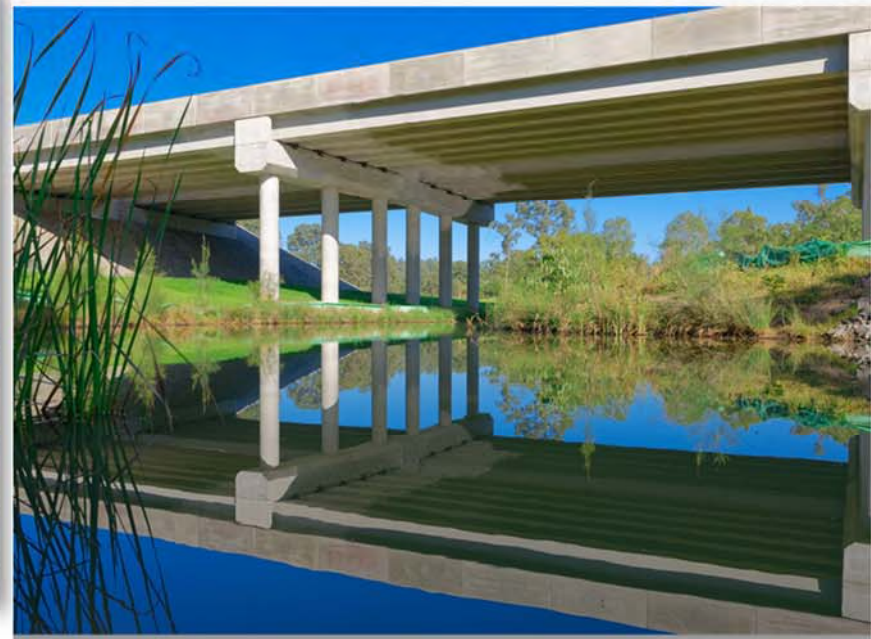
New Traveston Creek Bridge – fully rehabilitated creek bed with flowing realigned creek underneath
