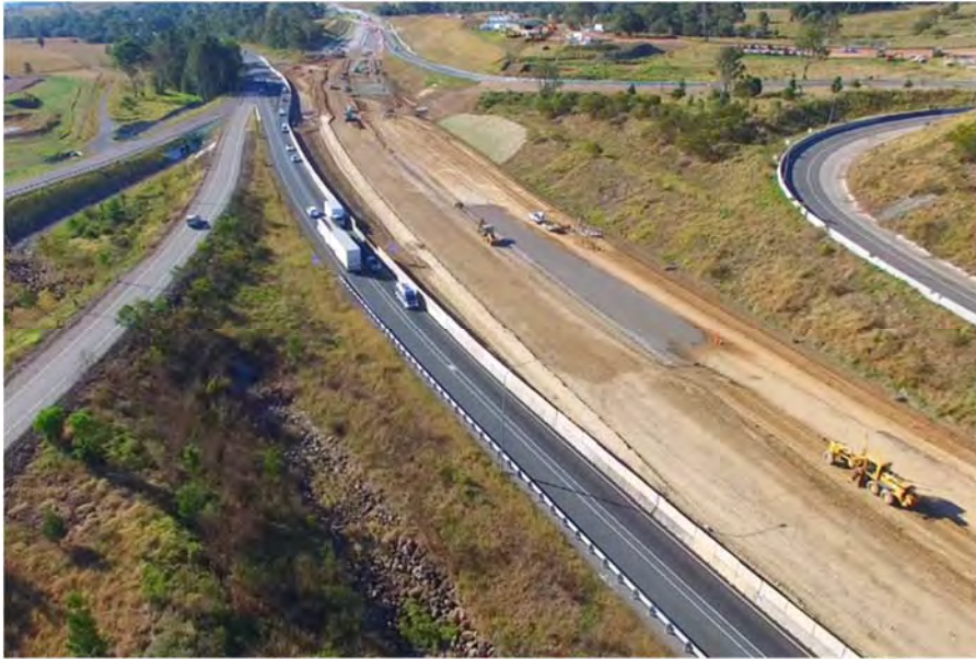
Tie-in at Traveston, where the existing Bruce Highway meets the new highway on the right (August 2017)
