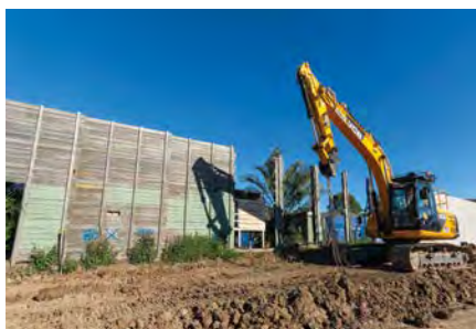
The existing noise wall at Bracken Ridge is being upgraded as part of the project.
