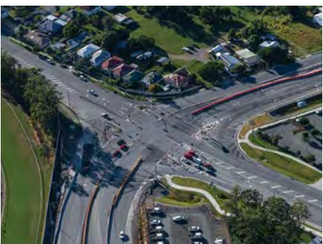
Depot Road/Braun Street/Board Street intersection upgrade is due for completion in late 2018.
