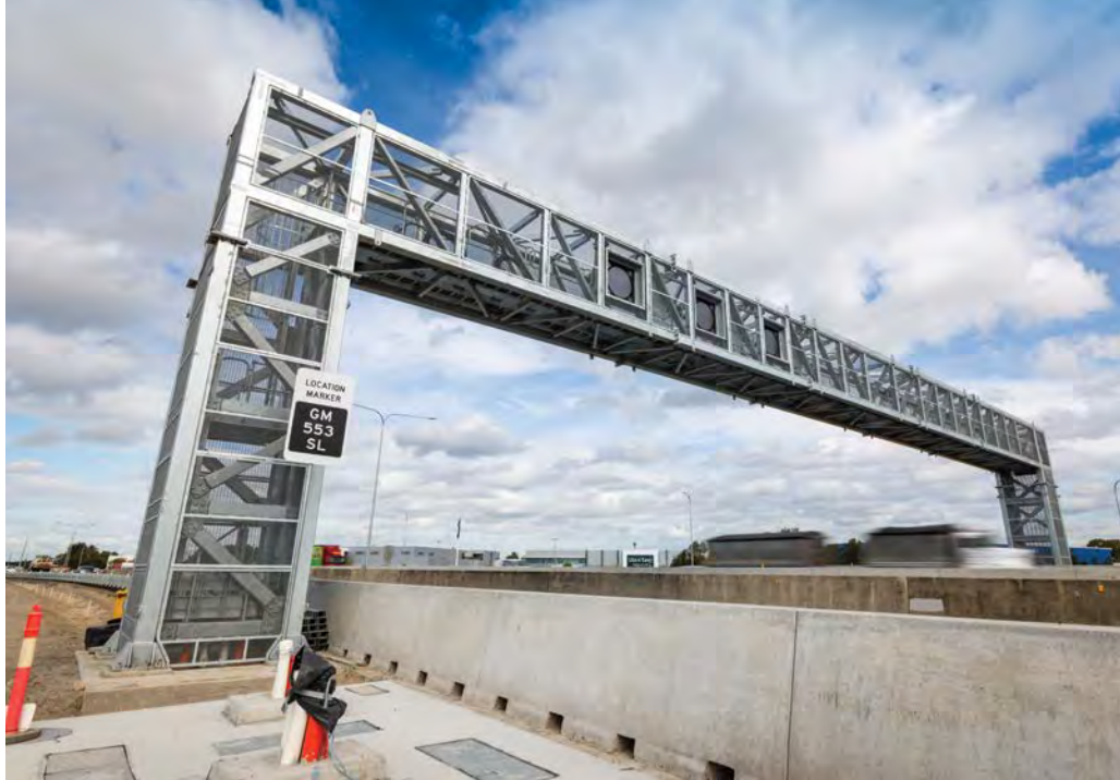
One of the new overhead gantries being installed over the motorway southbound lanes at Nudgee.
