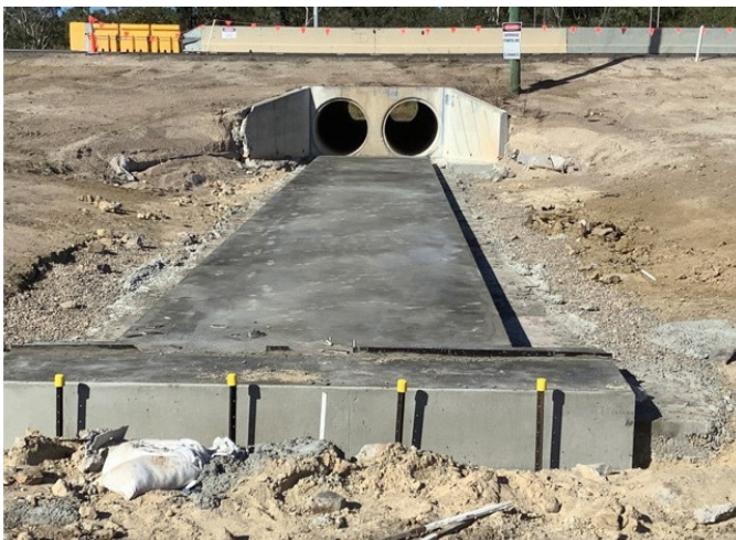
Culverts are being installed across the TNAIU project to compliment the natural water courses in the area
