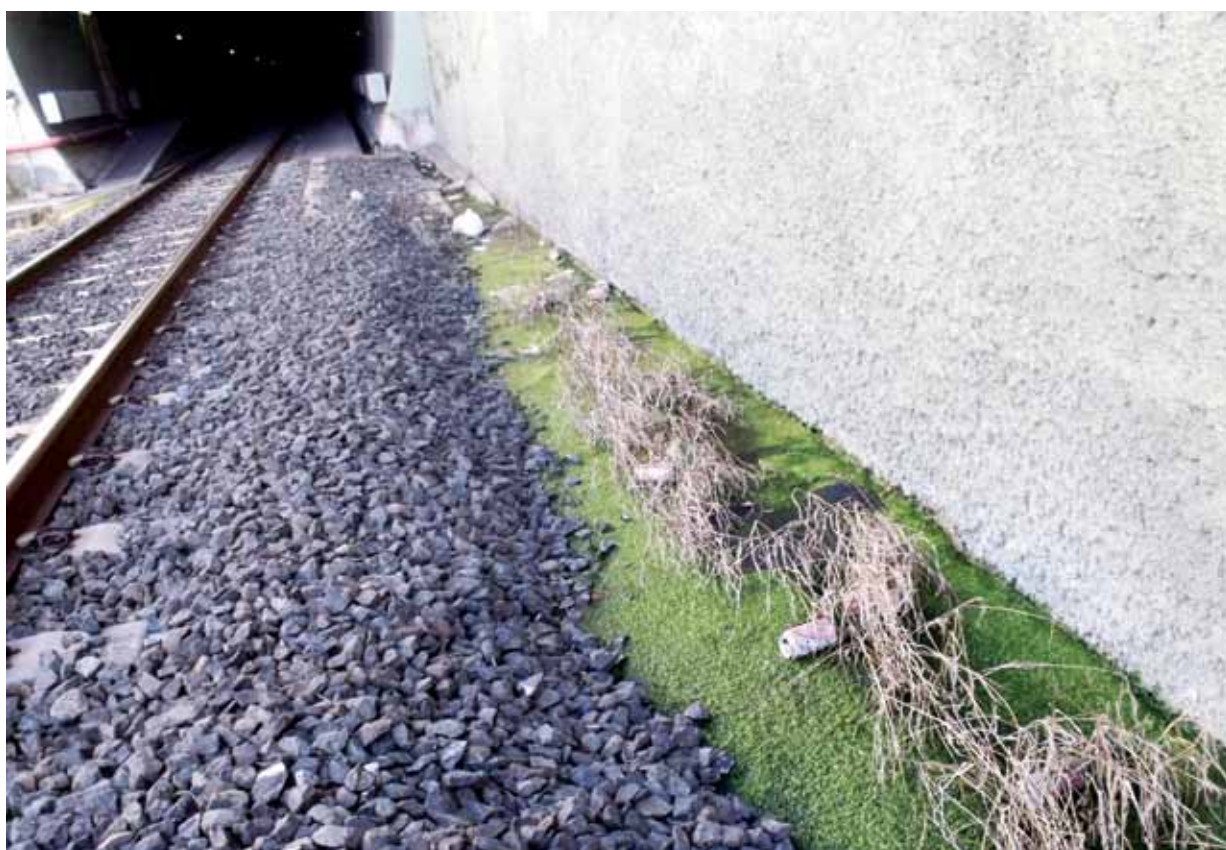
Figure B4 – Blocked drain at northern entrance to number 1 tunnel Fortitude Valley.
