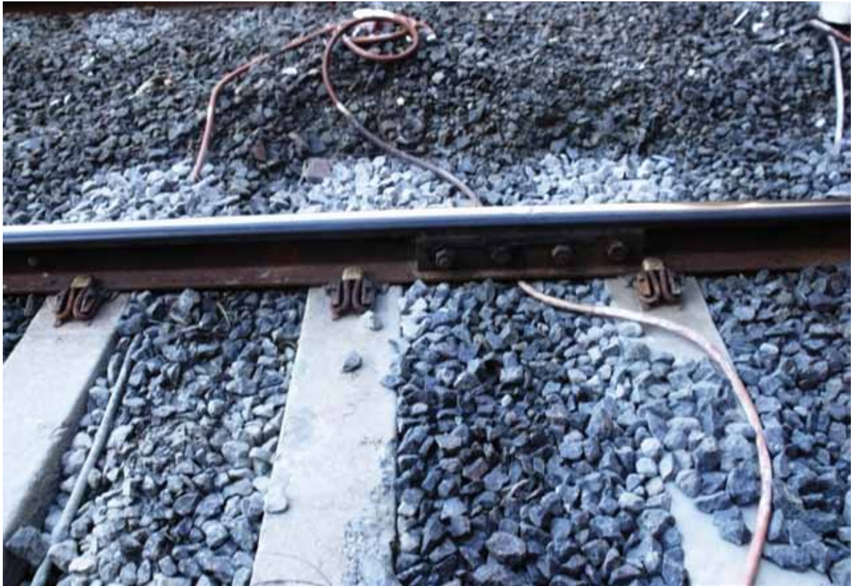
Figure B1 – Pumping sleepers (down main line between Fortitude Valley and Bowen Hills).
