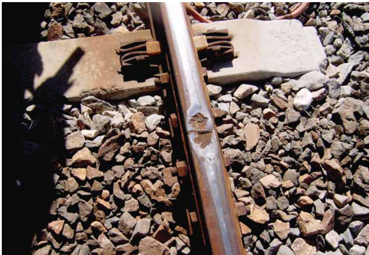
Figure B5 – Rail head damage on an insulated joint (down main line between Corinda and Sherwood). Photograph was taken on 15 May 2012 and the damage was repaired on 20 May 2012.
