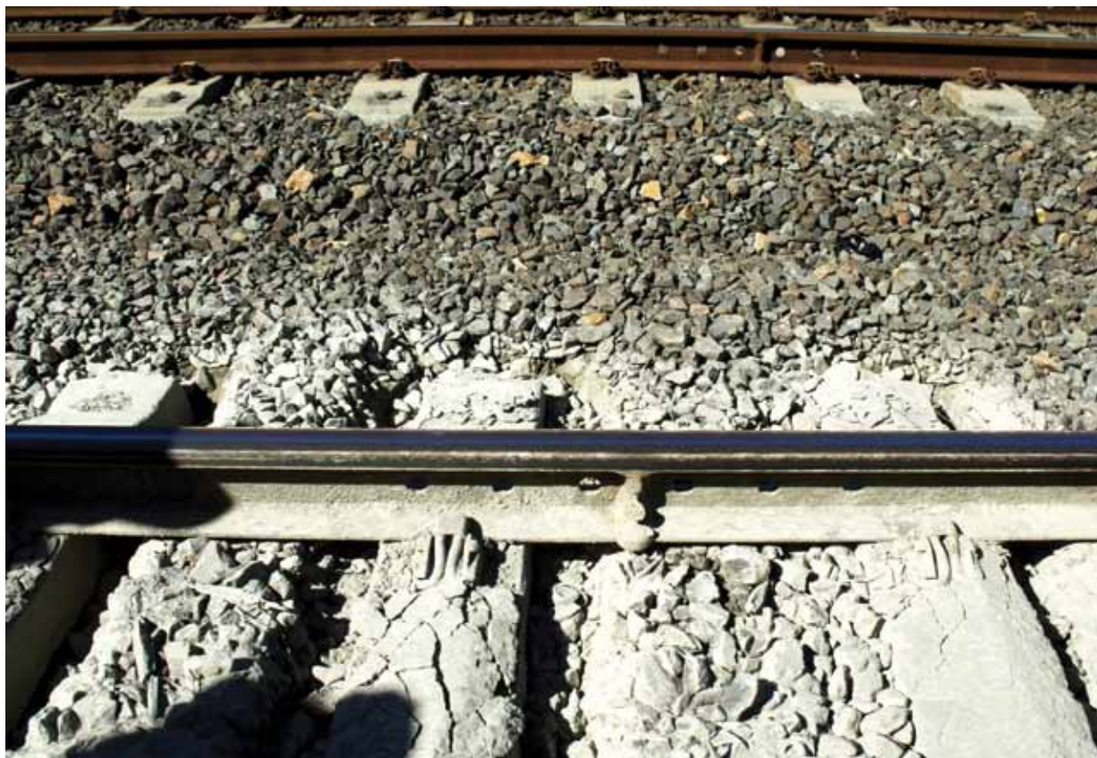
Figure B3 – Pumping sleepers and mud hole (down main line between Milton and Auchenflower).
