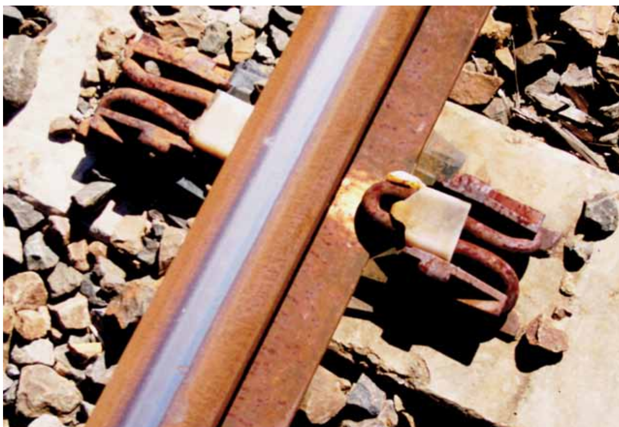
Figure B6 – Damaged rail fastening insulator (down main line between Corinda to Sherwood).
